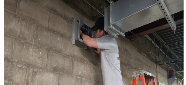
INSPECT FIRE DAMPER
