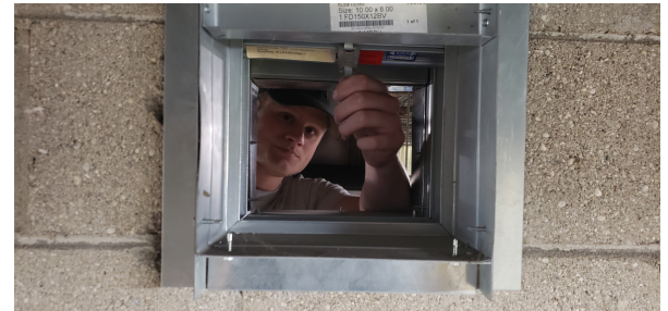
MAINTENANCE FIRE DAMPER
